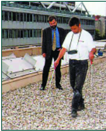
Figure 5: Leak detection procedure on an inverted BUR roof system. Locating breach through the ballast and insulation.
