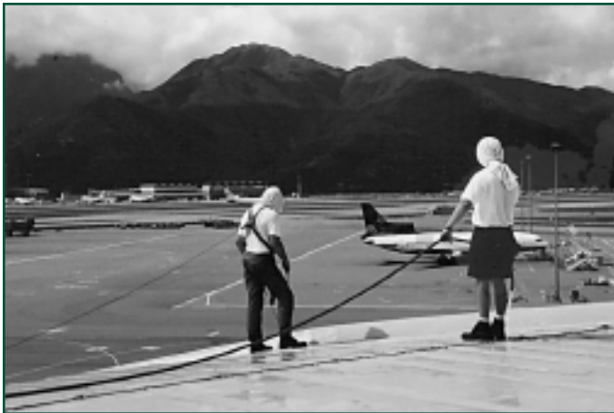
Figure 3: Leak detection at Chek Lap Kok airport, Hong Kong. Applying continuous flow of water on the sloped PVC membrane to facilitate the test.
