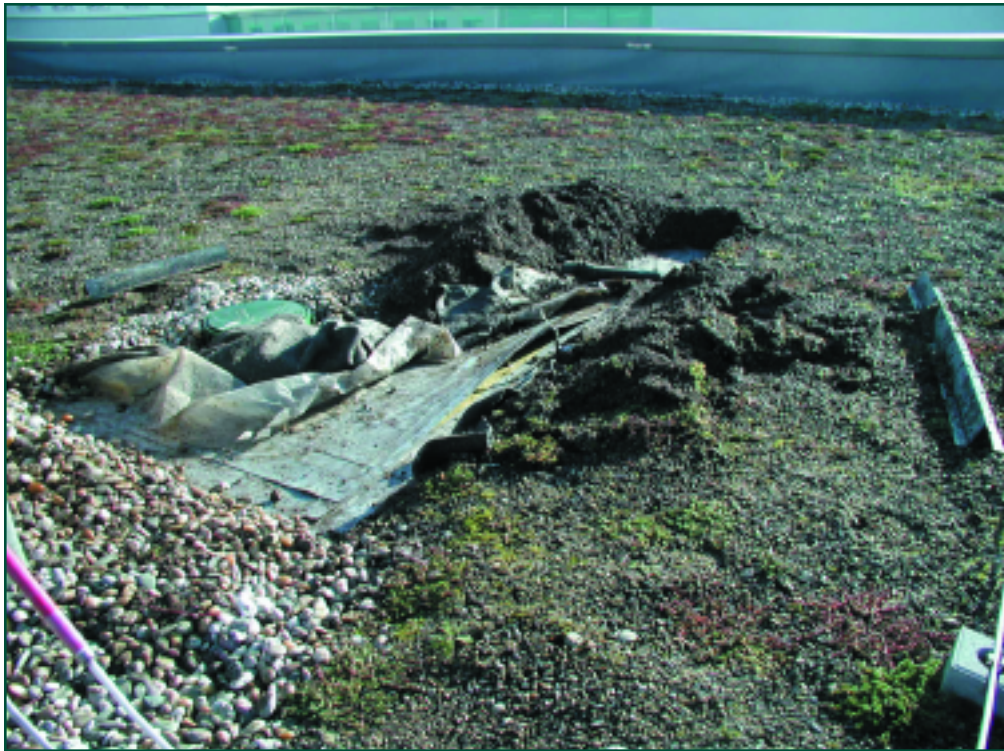
Figure 2: Leak investigation on a green roof in Frankfurt, Germany.
