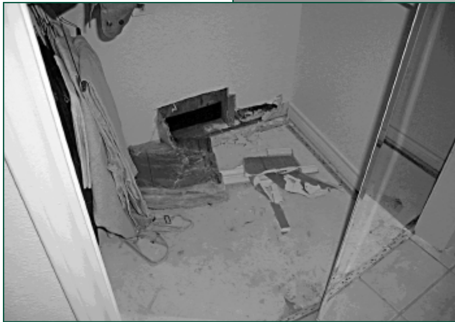
Figures 3-5: Interior water damage and organisms caused by inadequate flashing. Photos courtesy Norm L. Cooper, P.E.
