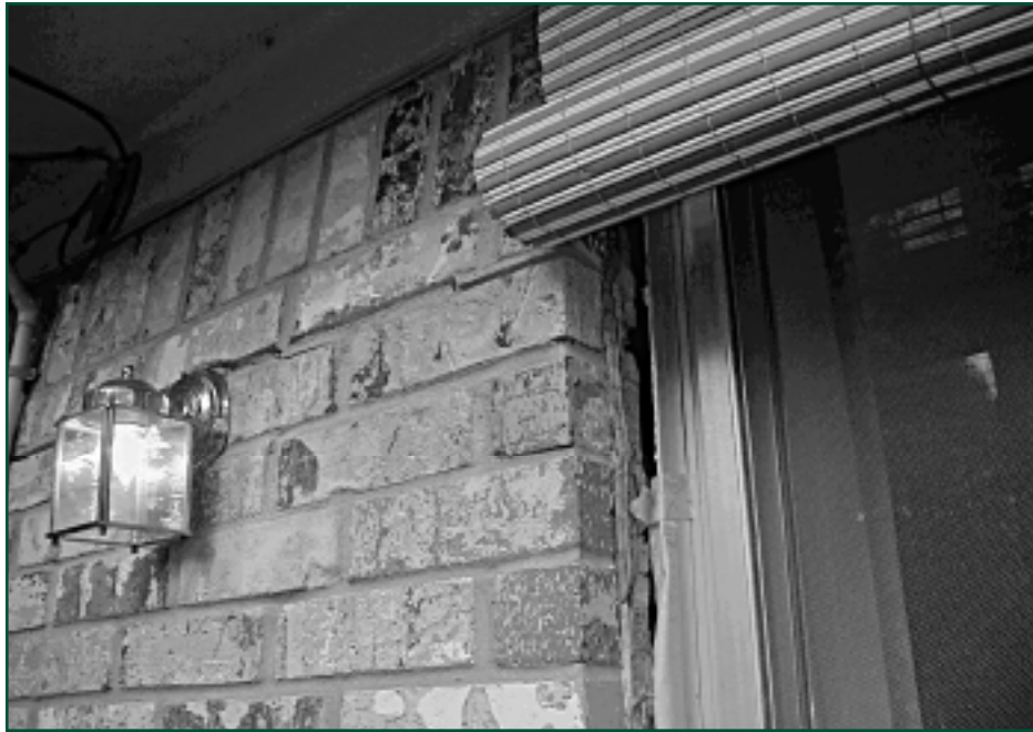
Figure 8: Inadequate metal ties between masonry and framing cause horizontal cracks, outward bowing, water entry, and risk of hazardous failure. Photo courtesy Norm L. Cooper, P.E.
