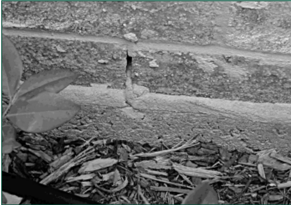
Figure 6: Blocked (or missing) weepholes cause water accumulation, rot, and hazardous spores. Photo courtesy Norm L. Cooper, P.E.
