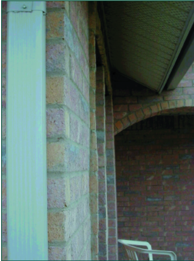
Figure 11: Brick misalignments out of tolerance. Photo courtesy Norm L. Cooper, P.E.
