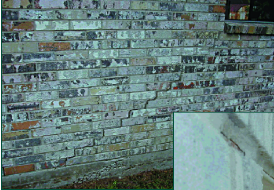
Figure 9: Inadequate drainage away from a building causes foundation movement, which causes brick (step) cracks. Photo courtesy Norm L. Cooper, P.E.
