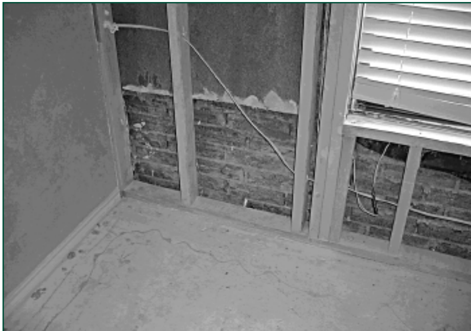
Figure 2: Missing and inadequate flashing behind brick siding caused leaks into a house, which caused hazardous spores. Photo courtesy Norm L. Cooper, P.E.
