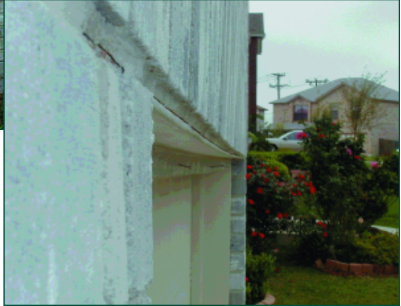
Figure 10: Inadequate and sagging door header causing brick cracks. Photo courtesy Norm L. Cooper, P.E.
