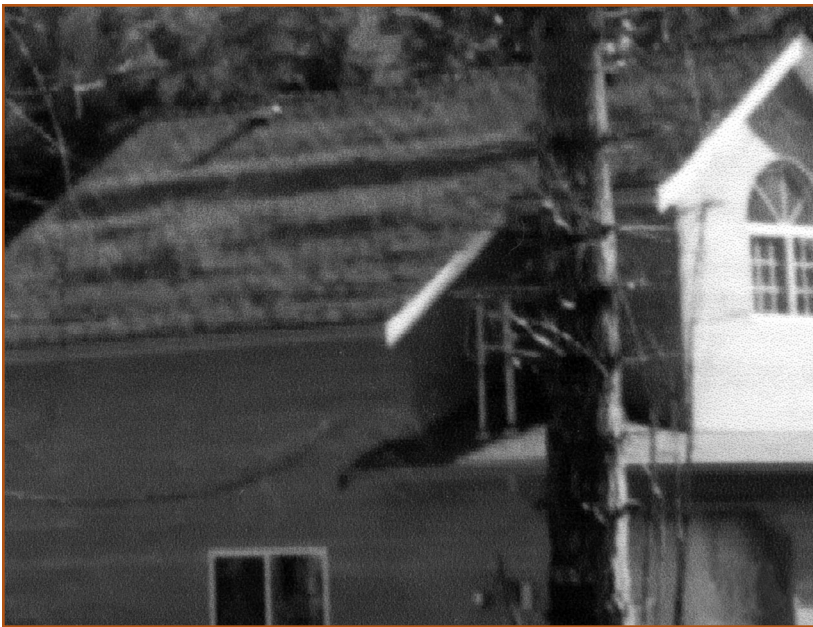
Photo 2: Severe sheathing distortion may be viewed on this unfinished home.
