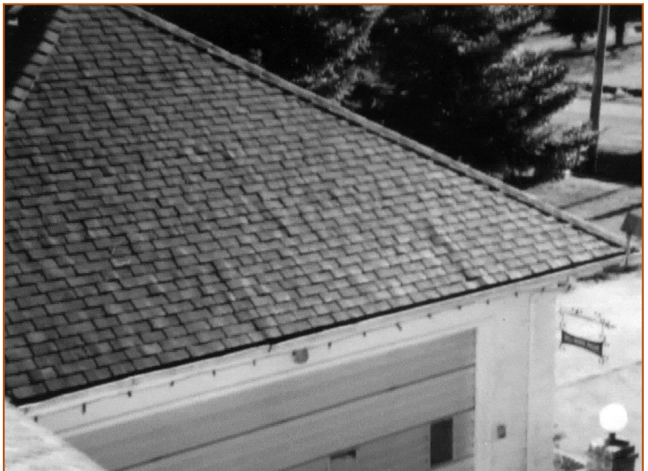
Photo 1: "Picture framing" buckles are obvious on this residence.
