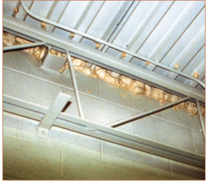
Where the steel deck runs perpendicular to the wall, two-component polyurethane foam is injected into the gaps between the steel deck flutes and into specially drilled holes in the deck itself in order to ensure continuity of the air barrier system.
