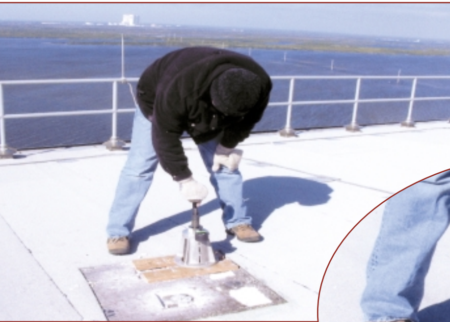
Left: Photo 16: Fastener Pull Out or Withdrawal Test conducted after removing the membrane and Dens-Deck, leaving the fasteners and 3" plates exposed.
