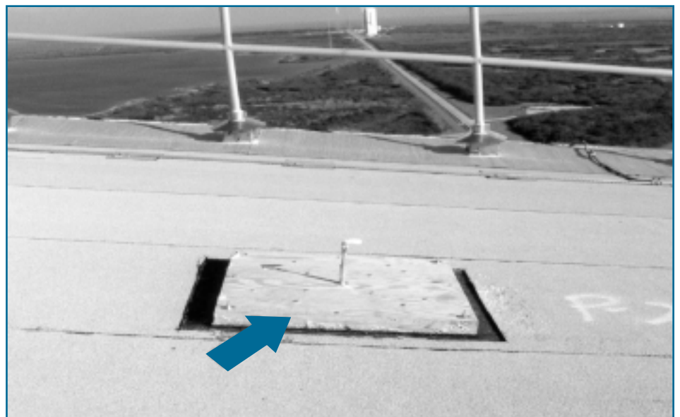
Below: Photo 13: Membrane trimmed away from edge of panel down to the top of the Dens-Deck. Eyebolt is in place and ready to attach pull device.
