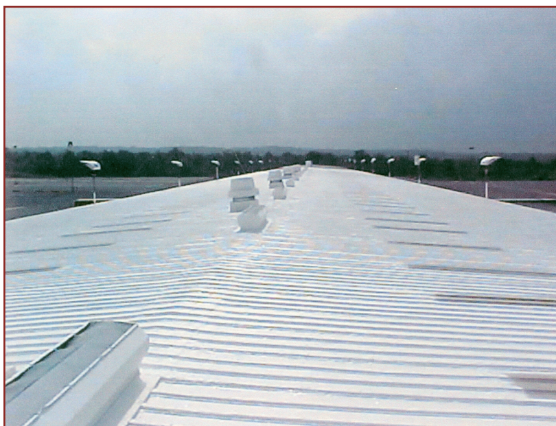
Metal roof restoration: before (top); sealing seams and fasteners (middle); and after (bottom).
