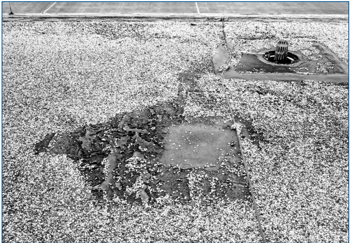
Photo 5: The repair to this roof system included removal of the loose aggregate surfacing. With the surface exposed, advanced deterioration of the organic felt is evident.
