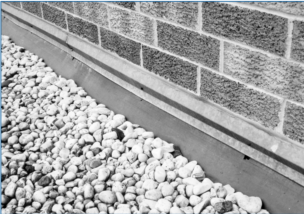
Photo 4: Severely bridging EPDM flashing is tearing away from the wall termination. A flashing replacement will prevent leaks and avoid a premature roof replacement.
