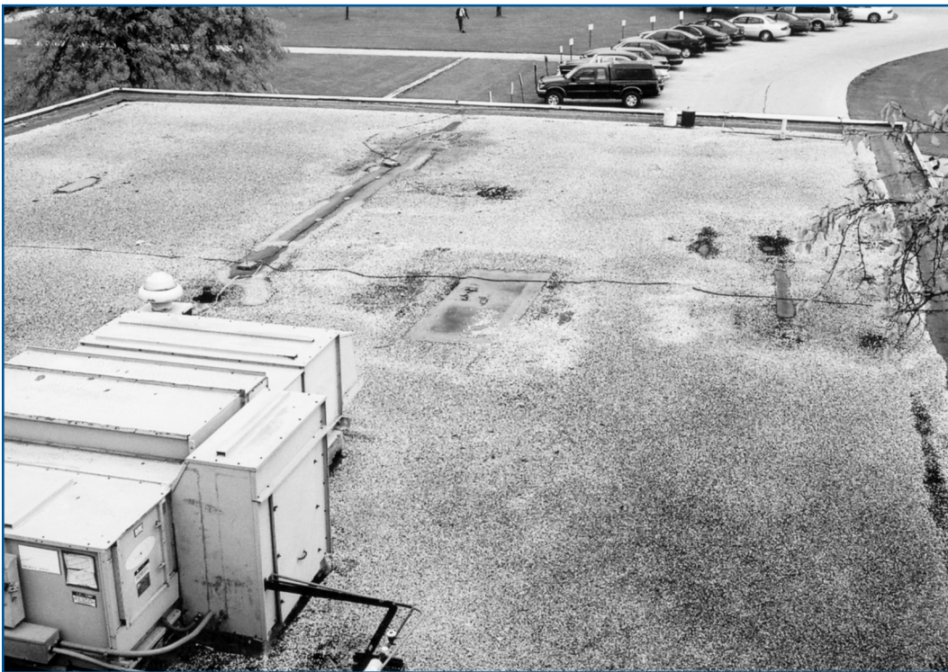
Photo 1: Overview of repairs made to a built-up roof system. These repairs are functioning, however, as the roof nears the end of its service life, additional repair work may not be economical.
