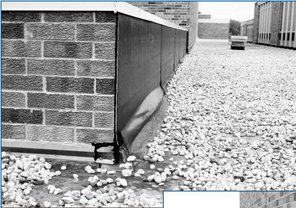
Photo 2: This severely bridging EPDM base flashing is a result of a termination failure. Installing new flashings on this 12-year-old roof system will provide several additional years of roof service life.
