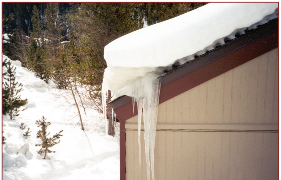
Figure 1: Typical ice dam formation at eave. Notice the eave is not even a substantial overhang.
