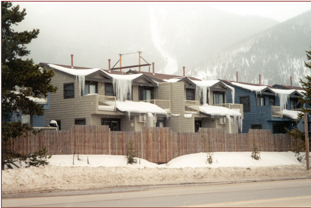
Figure 2: Severe ice dam formation along eaves and valleys.
