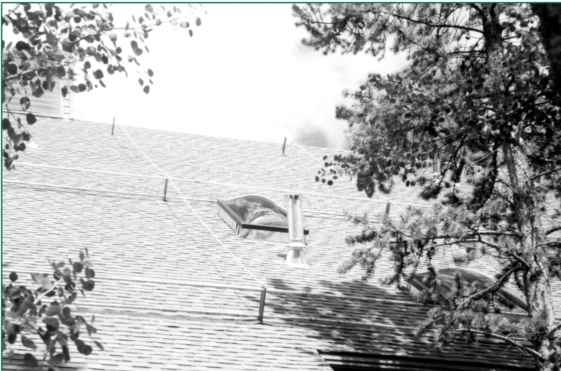
Figure 5: Snow fence and reinforcing cable system to retain snow on a 14:12 pitch roof.
