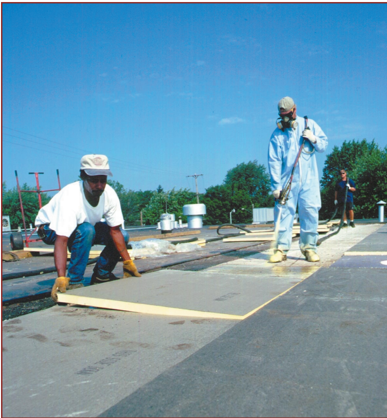
Insulation board stock being placed into a low-rise urethane adhesive (note 4 x 4 board size).
