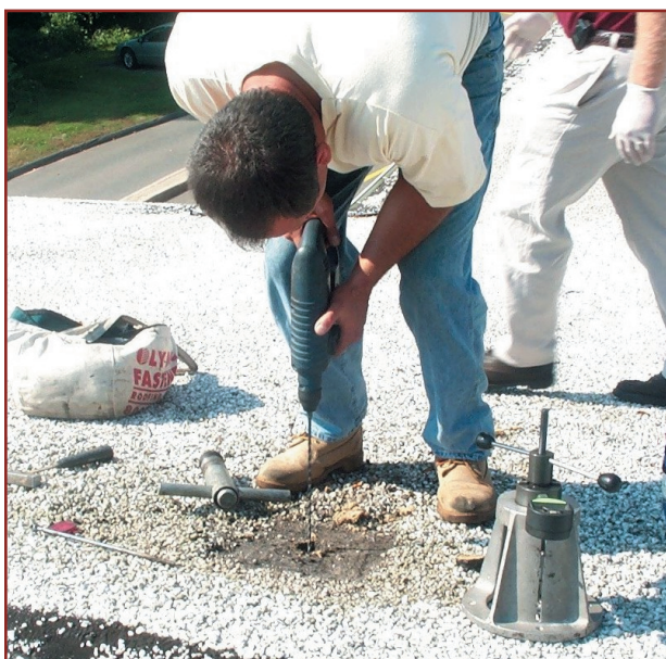
Technician predrilling a concrete deck before installing a fastener. Photo courtesy of Olympic Fasteners.
