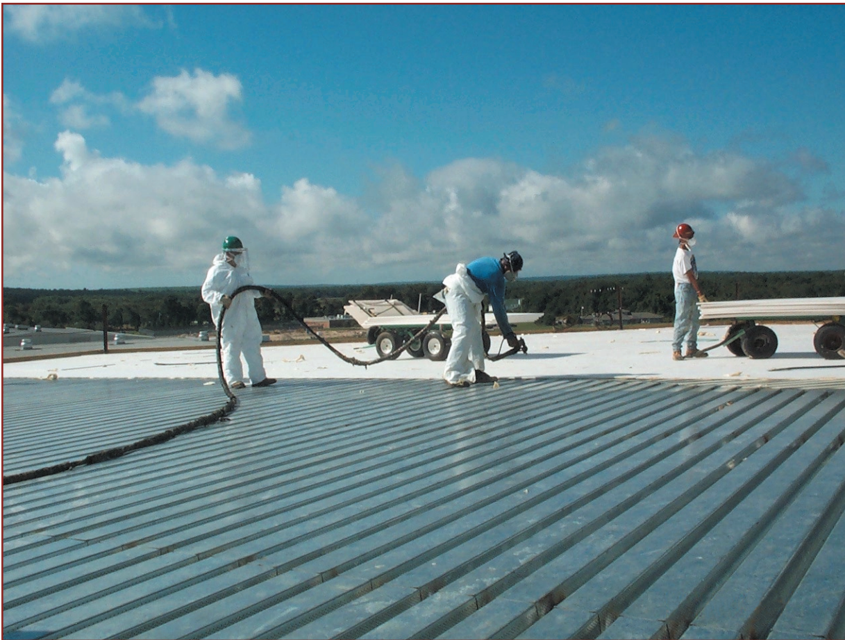
Contractor using a two-part urethane adhesive fastener where penetration of a mechanical fastener was unacceptable. Photo courtesy of Olympic Fasteners.
