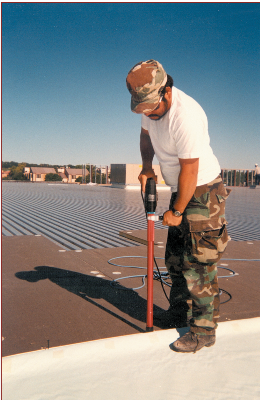
Contractor installing seam fasteners with a labor-saving and less tiring installation tool. Photo courtesy of Olympic Fasteners.
