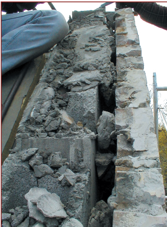
Photo 6: Cavity wall after limestone cap has been removed.
