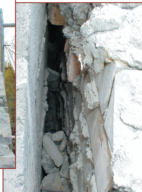
Photo 7: Closer view of cavity wall after limestone cap has been removed.
