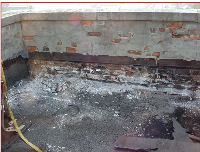
Photo 3: Parging with mortar coming off brick above metal counterflashing.
