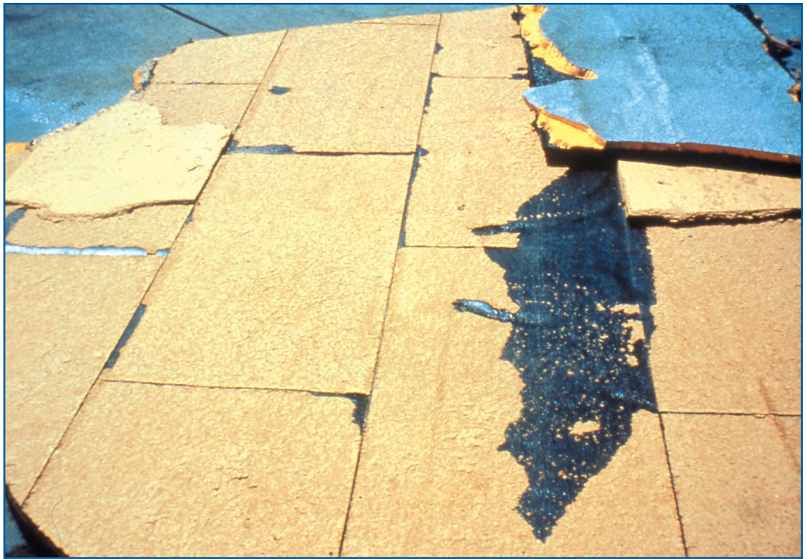
Delamination in the field of the roof may be the result of defects other than the edge.
