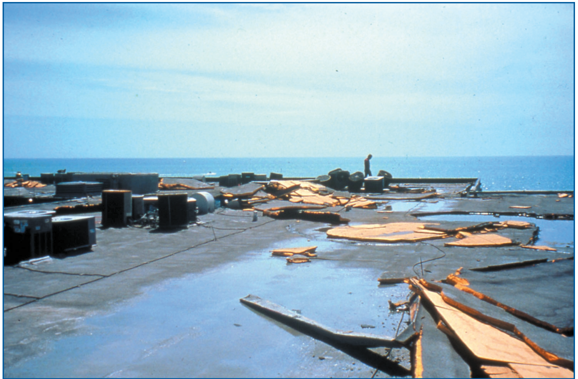
Wind damage can be very expensive.
