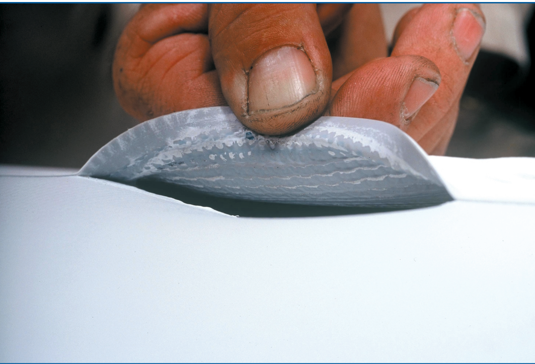
Photo 6: Delamination and membrane tear.
