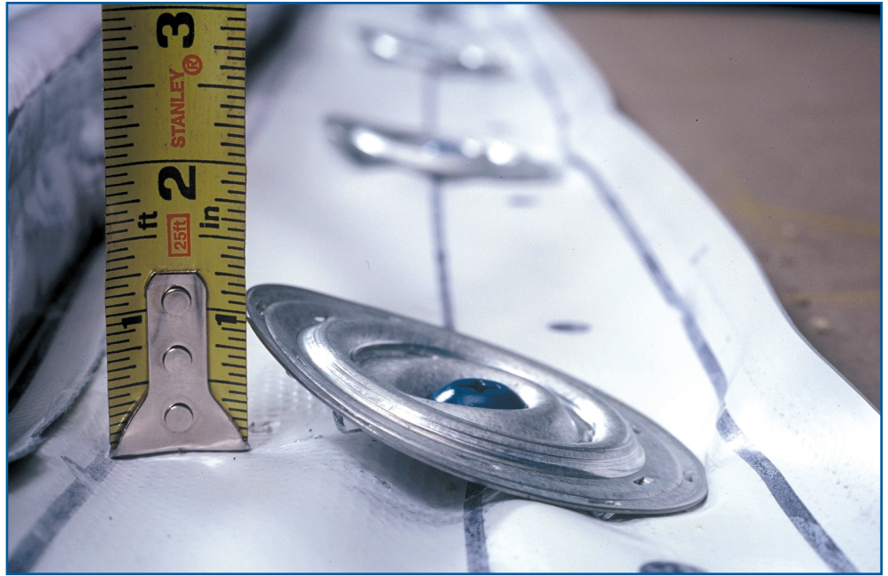
Photo 4: The 3-1/2"-round, 20-gauge metal plate is permanently deformed, as the membrane shows slippage and the fastener is rocking.
