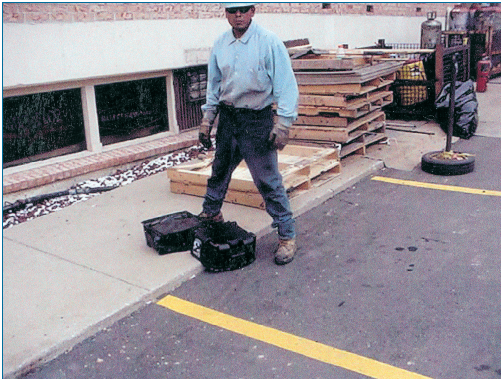
Photo 3: This worker for Hankins Roofing has just broken a 60-pound package of low-foaming asphalt into two 30-pound blocks.
