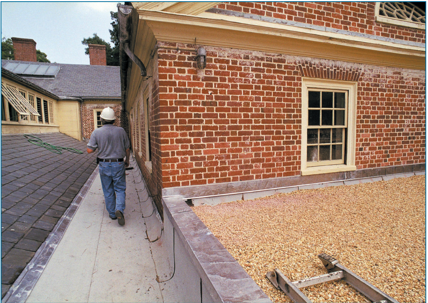
Photo 2: Gary Ramsburg of Roof Engineering Corp., Norfolk, VA, walks along the gravel surface of the BUR system his firm installed on The Inn at Colonial Williamsburg.
