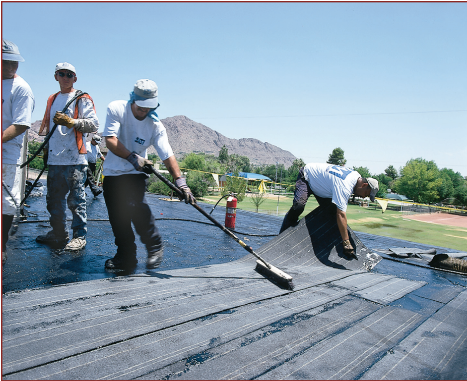
Brooming to ensure full adhesion of the BUR felt and respective plies.
