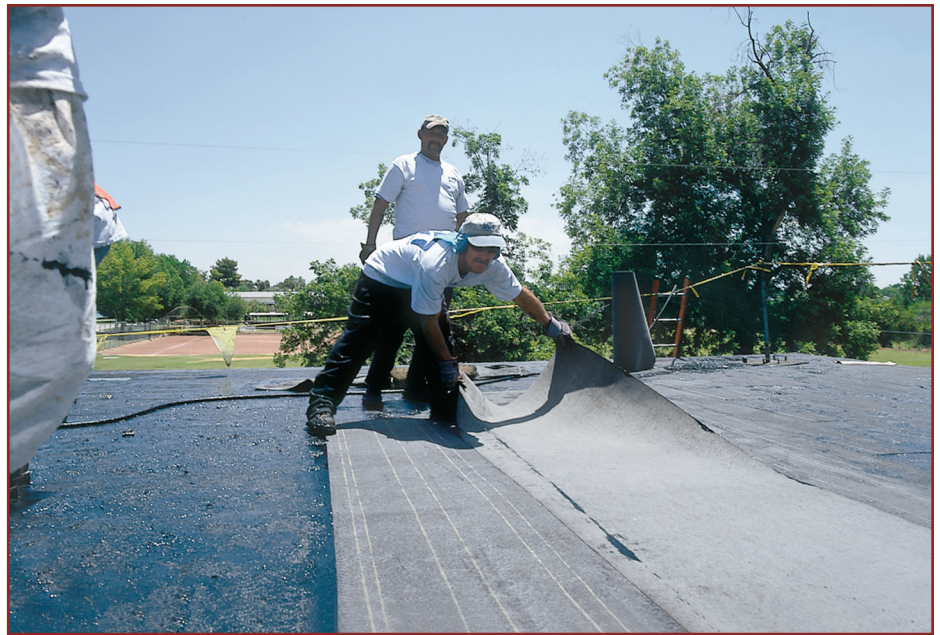
Roofers laying the cap sheet in cold adhesive using the mop and flop method.
