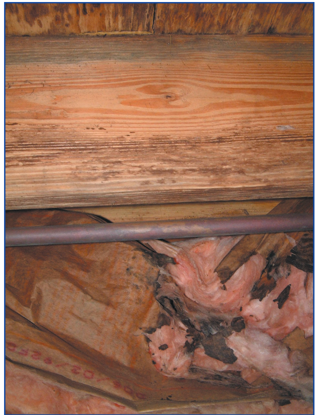
Figure 6: This photograph is interesting, as it shows both types of damage on one floor joist. Damage extends approximately one-third of the width of the board from the top and bottom. The middle third of the joist is bright, yellow, and free of visible damage.
