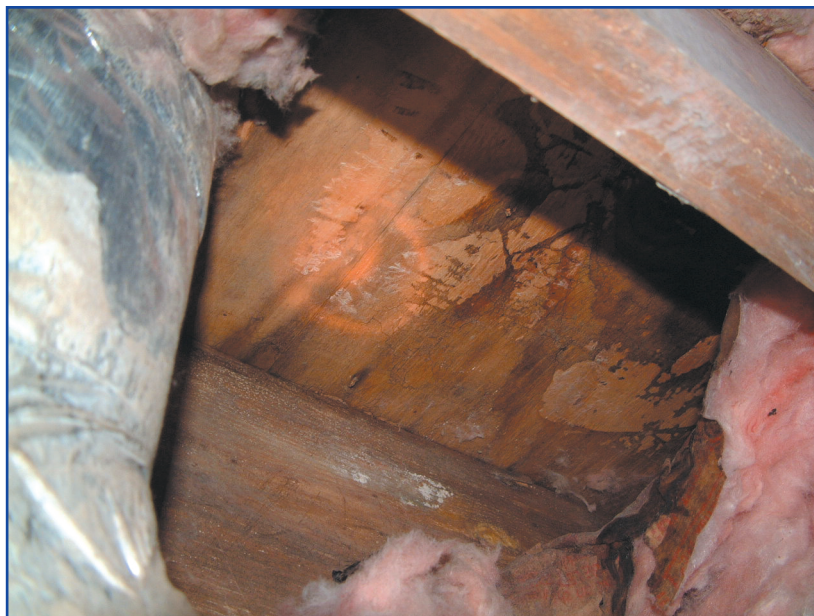
Figure 5: The second type of moisture damage starts at the floor sheathing and migrates downward. This type of damage is associated with excessively cool interior floor temperatures and low permeability floor finishes. This photograph shows a section of flooring near a "toe-space" HVAC register where supply air discharges horizontally from below a cabinet.
