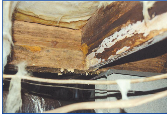
Figure 4: Left unchecked, crawl spaces can suffer high severity moisture-related damages. The floor framing in this Georgia home partially collapsed during a holiday dinner party. Wood-destroying fungi compromised the strength of the wood members to such an extent that they could not support design level loads.
