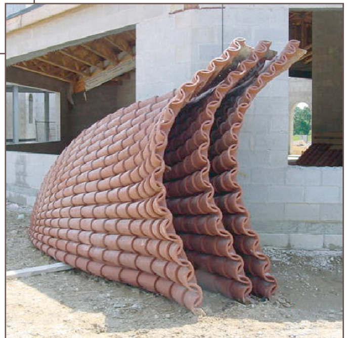
Figure 8 - Outer domes were fabricated and delivered to the site in pie-shaped segments.
