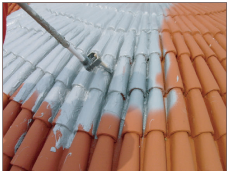
Figure 15 - Application of the elastomeric base coat in all the crevices with a brush.
