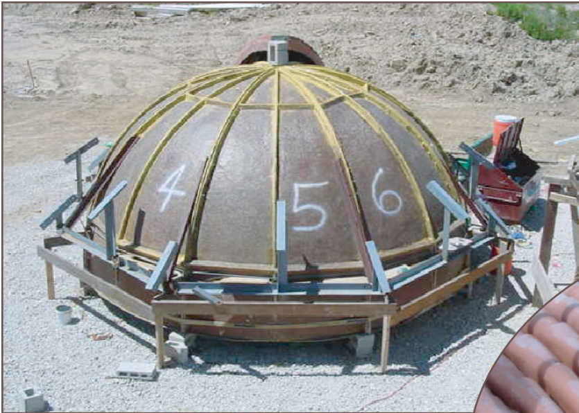
Above: Figure 9 - An inner dome being assembled on the structural steel skeleton.
