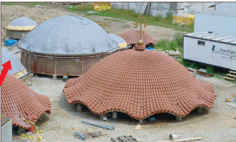
Above: Figure 11 - Assembled inner and outer dome. Note the gray spray polyurethane foam system and the perimeter drain pipes (red arrow).
