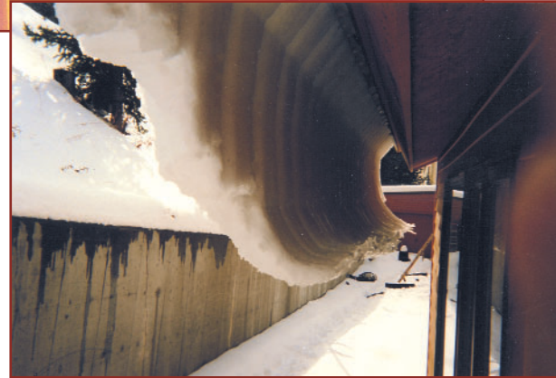
Snow and ice sliding off metal roof and curling into window.
