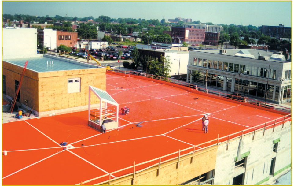
Photo 4: Lucas County Public Library, Toledo, Ohio. Photo, courtesy of Midland Engineering, South Bend, Indiana.
