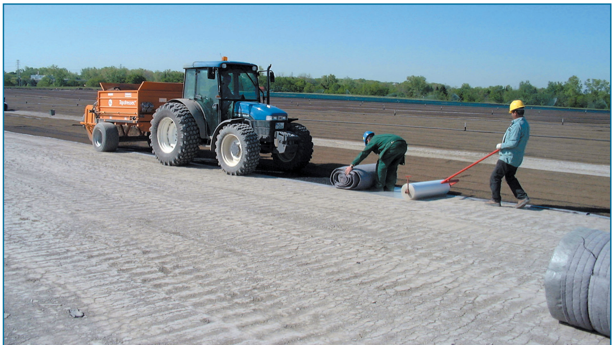
Figure 4: Procedure for applying polyethylene root barrier, vegetation mat, and substrate sequentially at cultivation site in Allen Park.
