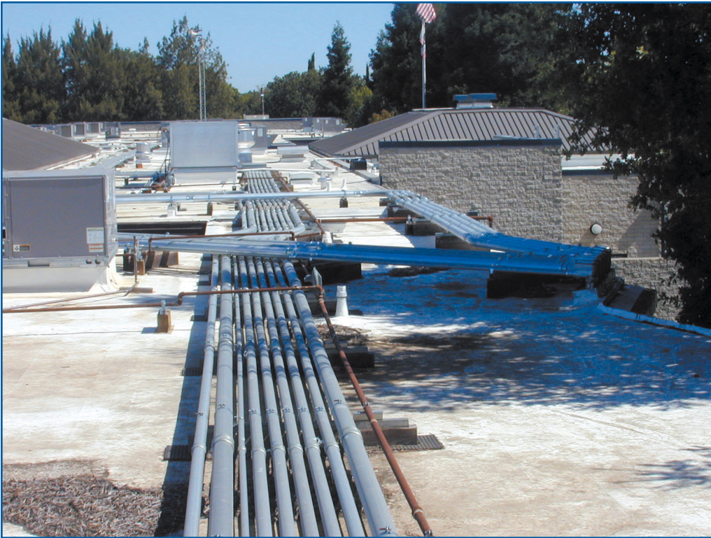
Numerous pipes would present a problem to either tape or GPS. Capabilities were added to collect pipe features by recording the centerline and adding the number of pipes.
