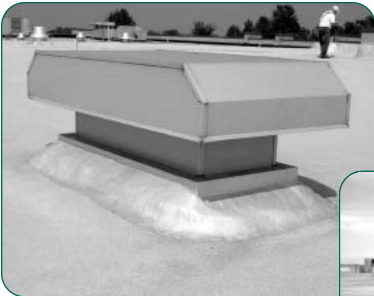
Figure 9 - Equipment support – high curb.
