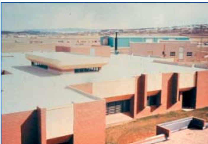
Typical SPF roof.
