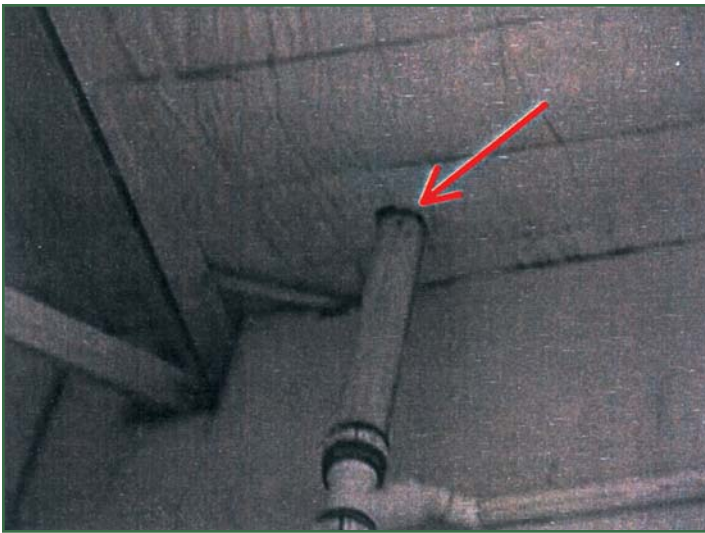
Photo 6: Insulation facer is not sealed around projection through roof.
