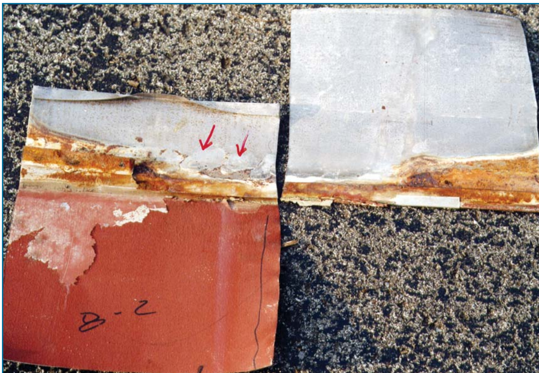
Figure 10: The left panel is the down-slope panel. The arrows indicate solder that was used to attach the lock-strip. Both sides of the lock-strip were very corroded. The right panel is the underside of the up-slope panel.
