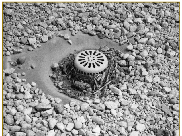
The roof drain shown here is dangerously clogged with debris, an all-too-common condition.
