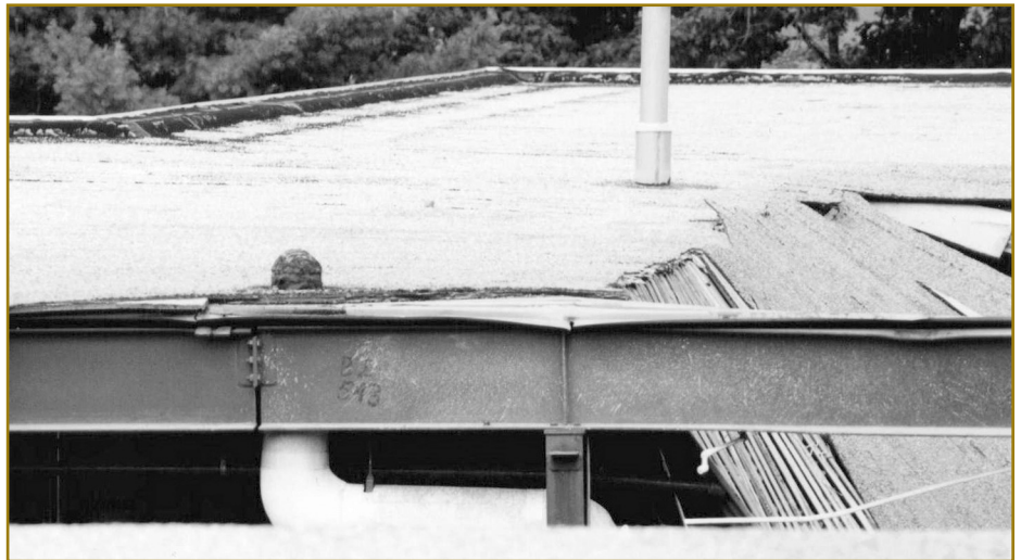
This photo shows a partial roof collapse from excessive weight of ponded water due to a clogged drain strainer.
