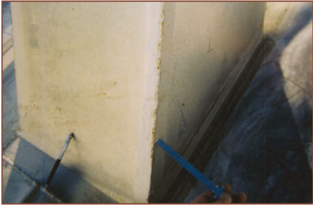
This Galvalume curb (left) was shop welded, resulting in traces of red rust at the vertical edge of the curb after just one year.
