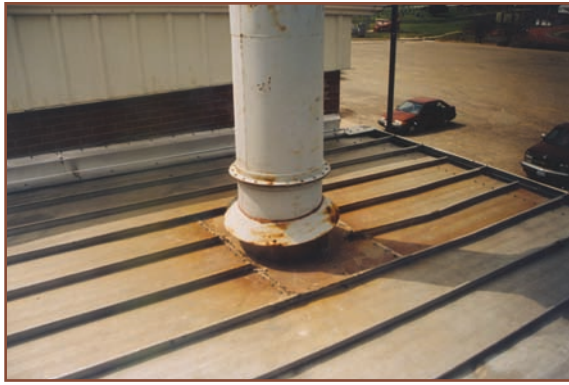
Exhaust flues that discharge gases from burning fossil fuels can cause a micro-acid rain environment near the flue.
