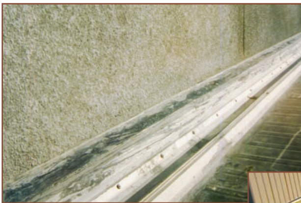
Alkali in the mortar from this stucco wall (far left) induced corrosion of the Galvalume. The black stain is accelerated oxidation of the aluminum.
