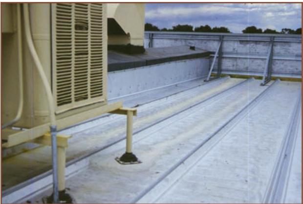
Dripping from a rooftop unit can cause corrosion as shown on this 1-1/2-year-old roof. In another year and a half, the white zinc oxide trails will turn red with iron oxide.
