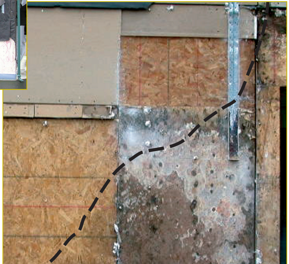
Photo 2 - Hardwood OSB sheathing with severe white-rot decay is surrounded by relatively undamaged hardwood OSB. The dashed line traces the upper limit of the migrating water. Note that the white-rot deterioration has spread upward from the water line. (The localized brown-rot decay at the upper right is spreading from underlying infestation of a softwood-framing member.)
