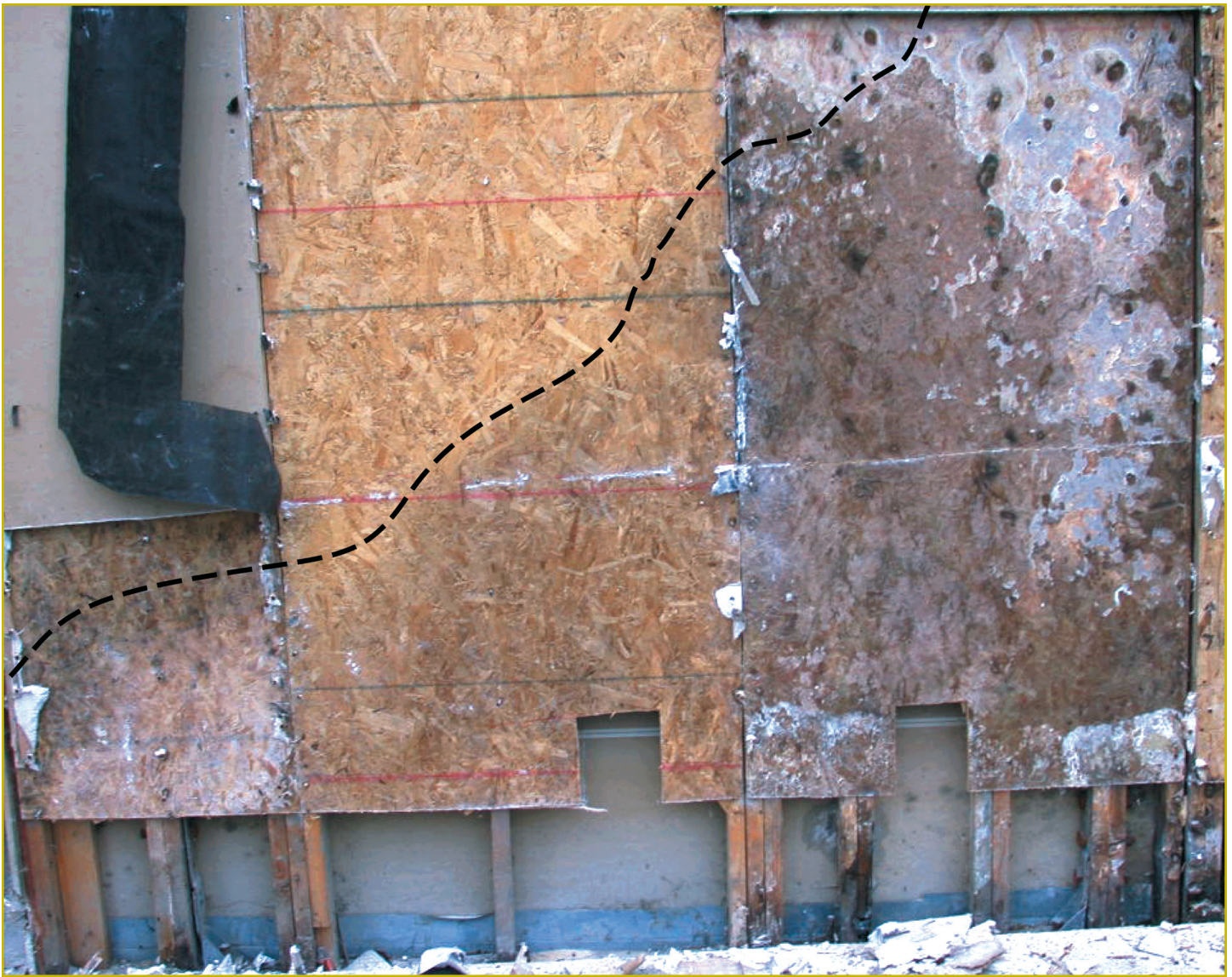
Photo 3 - Undamaged center panel is sandwiched by two white-rotted panels. (The dashed line traces the upper limit of the migrating water.)
