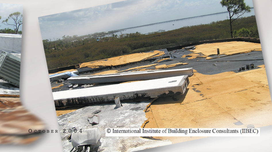
All from the same location—Below left: BUR and SPF blown off phenolic foam insulation. Directly below: BUR with SPF surface blow off. Below right: Hollow core concrete deck blow off.
