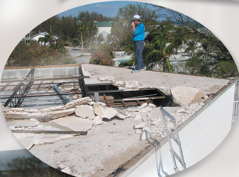
Above: Sanibel Island BUR blow off. Left: This single-ply, only 500 yards from the photo above, survived.
