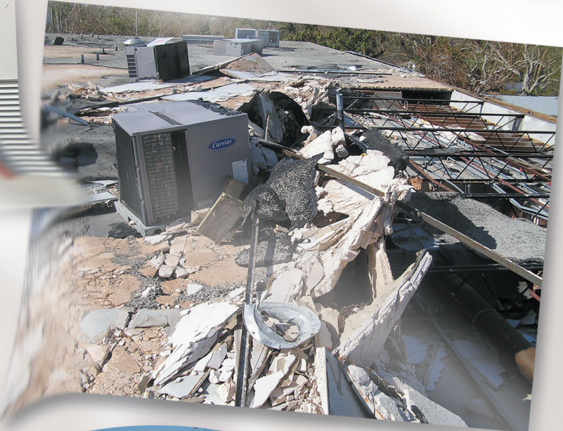
Left: Wood truss and deck with metal roof blow off at the Charlotte County Fire Station 12 in Punta Gorda. Below: Extensive deck loss on built-up roof on Sanibel Island.
