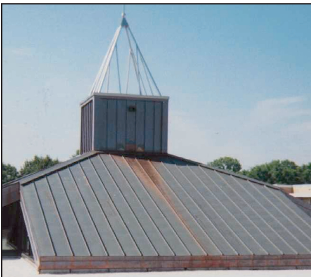
Figure 5: Uneven weathering caused by the flow of rainwater from an asphaltic-based roof covering onto standing seam copper.
