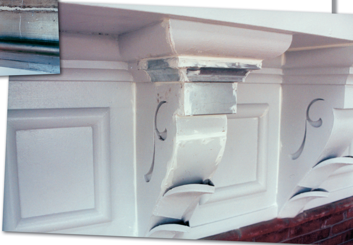
Below: A typical in situ repair of a retained corbel at the main building cornice.
