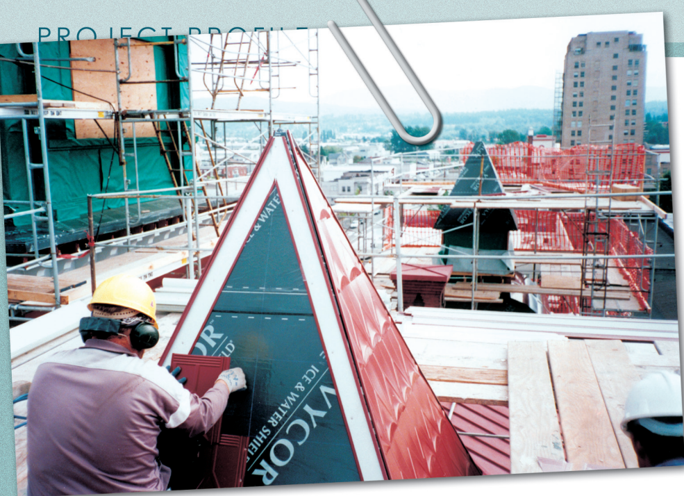
The foreground cupola is being shingled, while the background cupola has only the self-adhering waterproofing underlayment in place and breathable underlayment is being installed at the central clock tower.
