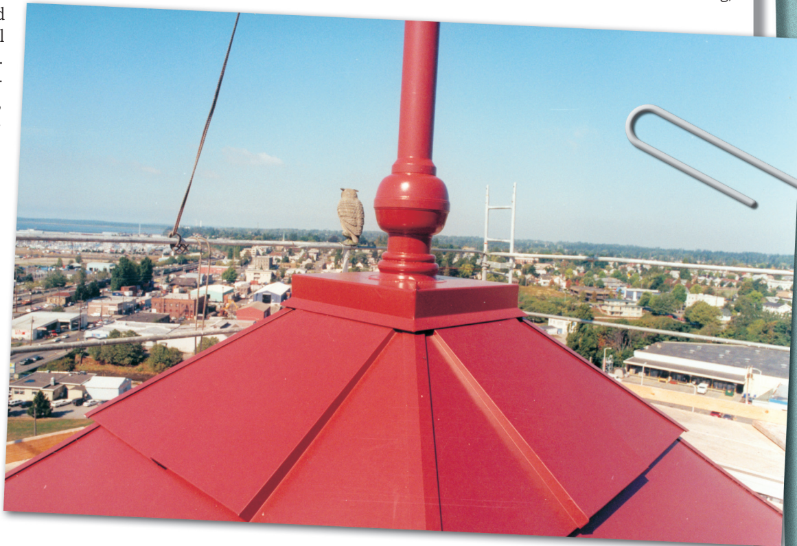
A particular highlight of the work was the completion of the uppermost Bermuda-style roof with its raised central panels that caps the central clock tower.
