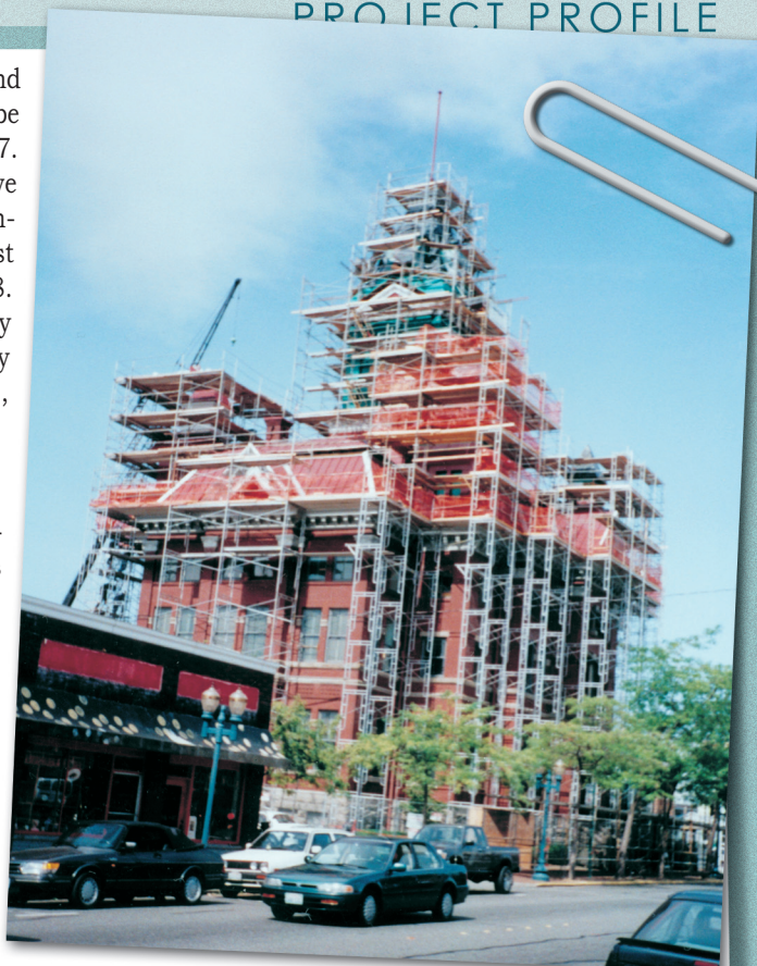
Although some work on the building envelope occurred below the roof line at the main building cornice, full scaffolding was erected, primarily for the replacement of the roof.
