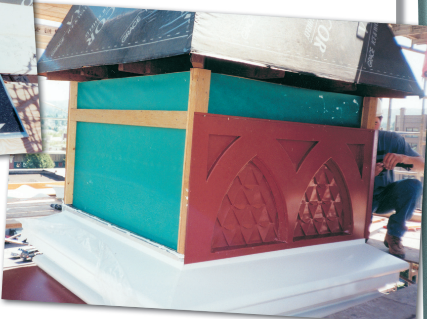
Right: "Fish scale" panels are being reinstalled at the northeast cupola with new wood blocking at panel perimeters. Note the use of breathable underlayment at the cupola wall and waterproofing underlayment at the pyramidal hipped roof above.
