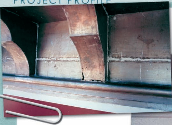
Left: Where paint removal revealed deteriorated metal where decorative sheet metal had been intended for retention, the sheet metal was repaired in situ.
