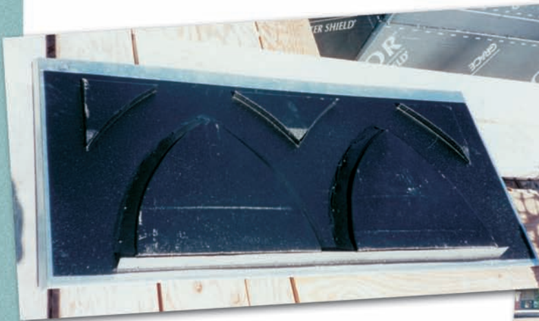
Above: The back side of a cupola "fish scale" panel reveals the polyurea resin coating that was applied to stabilize the panel. In addition, the panel edges were reinforced with galvanized steel formed angles.
