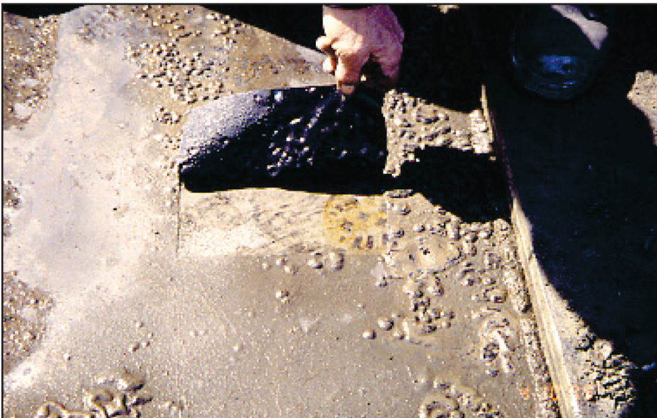
Figure 7: Delamination of liquid-applied membrane
