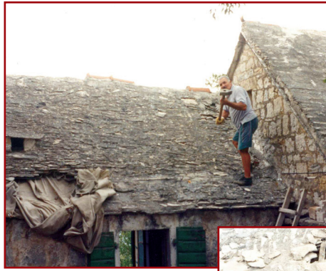
Figures 6a and 6b: Beginning of work; taking stone tiles down from the roof.
