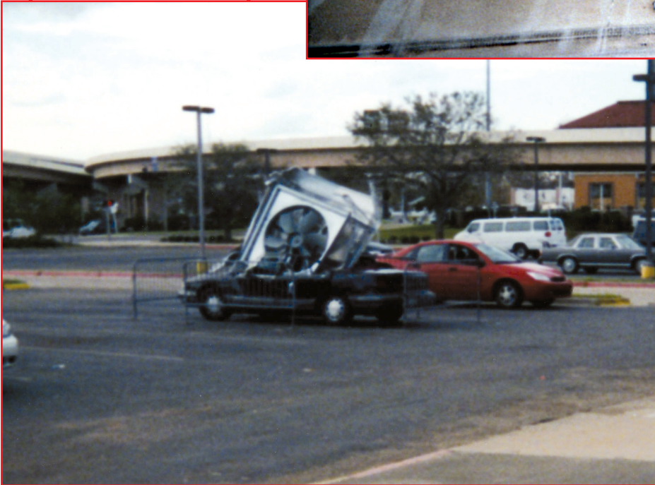
Photo 3: Exhaust unit blown off the roof.
