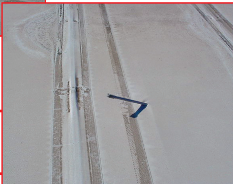
Photo 5: Membrane punctured by an exhaust unit.
