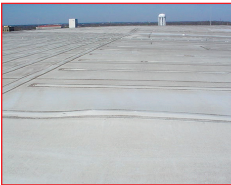
Photo 7: Partially deformed fixation bar.
