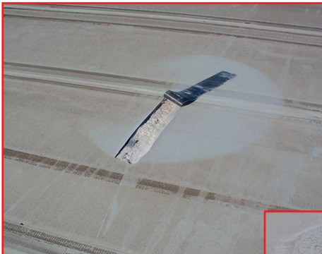
Photo 4: Membrane cut by an exhaust unit.
