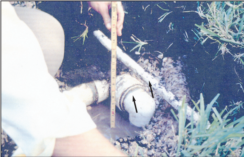
Figure 4: Elevated drainage pipes.
