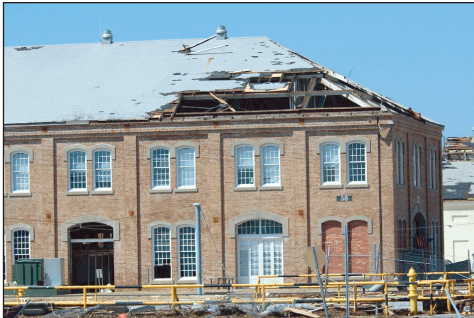
Figure 2: Damage caused by Hurricane Ivan on the Florida panhandle.
