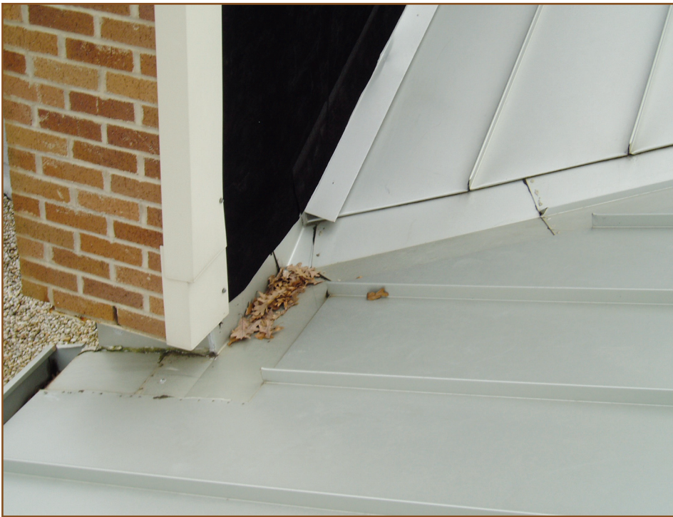
Photo 2 – Improper valley detail and termination.
