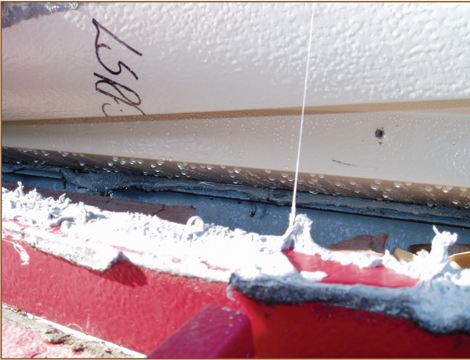
Photo 4 – Significant condensation within ridge cap.
