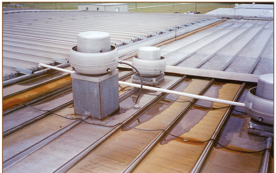
Photo 3 – Classic improper penetration flashing.
