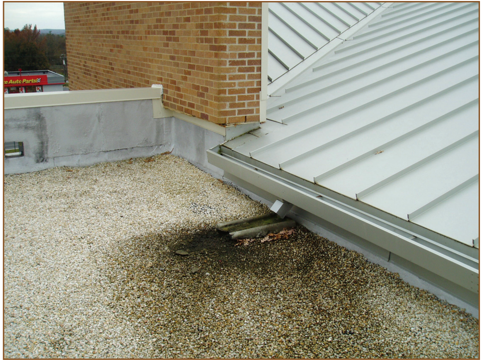
Photo 1 – Drainage deficiency on a one-year-old project.
