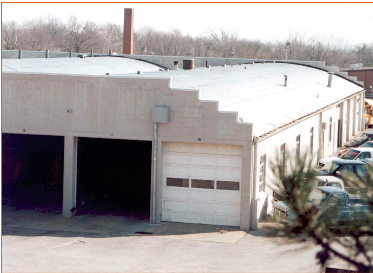
Adjacent curved roofs create valleys for moisture infiltration and parapet wall problems.
