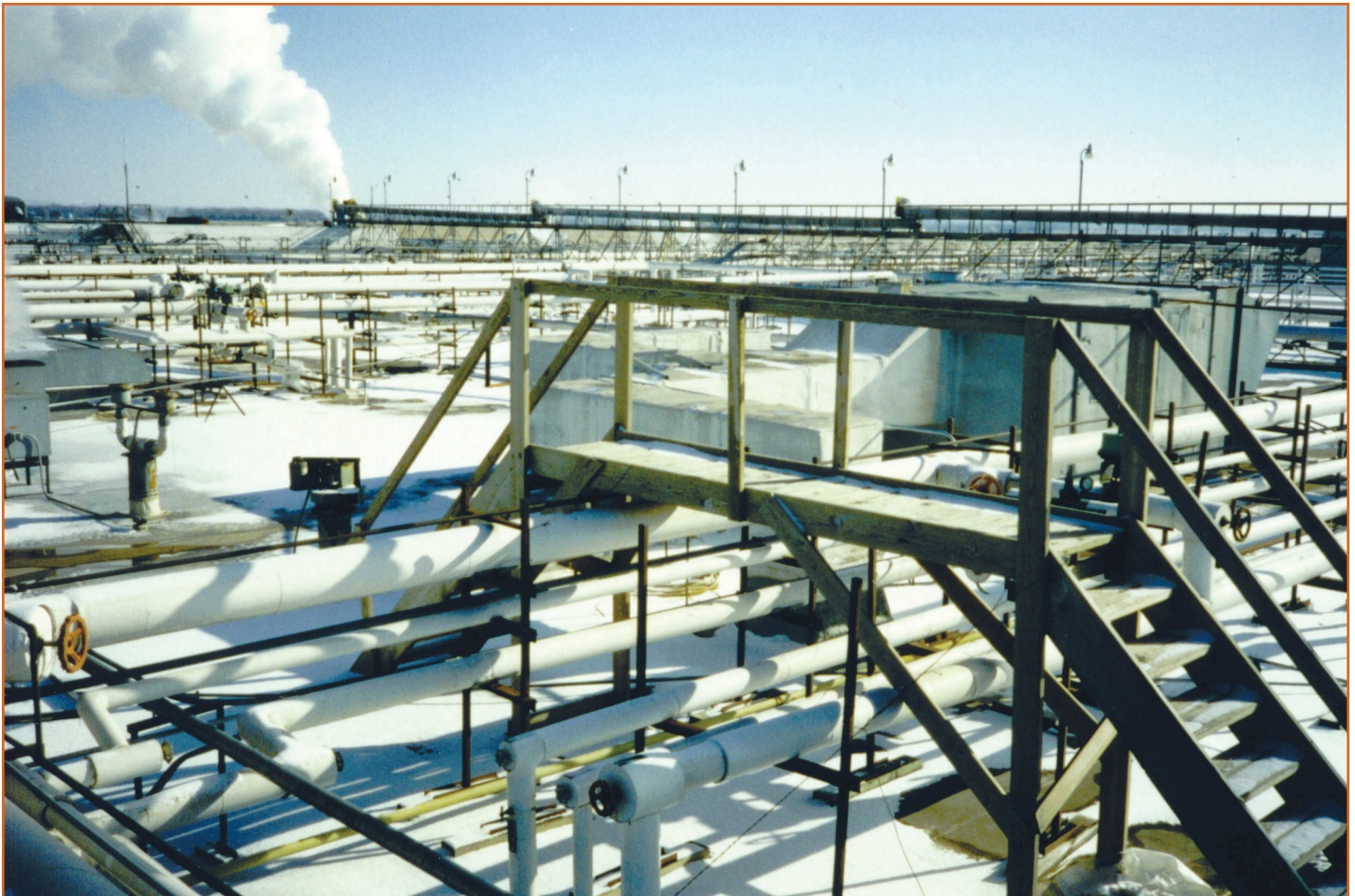
The roof of a beef processing plant with numerous roof penetrations and obstructions.
