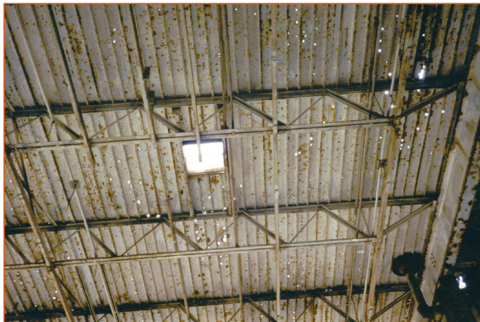
This steel roof deck has numerous holes created by severe corrosion.
