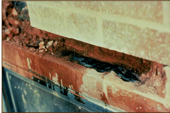
Figure 5 – Water runs around end of concealed flashing.
