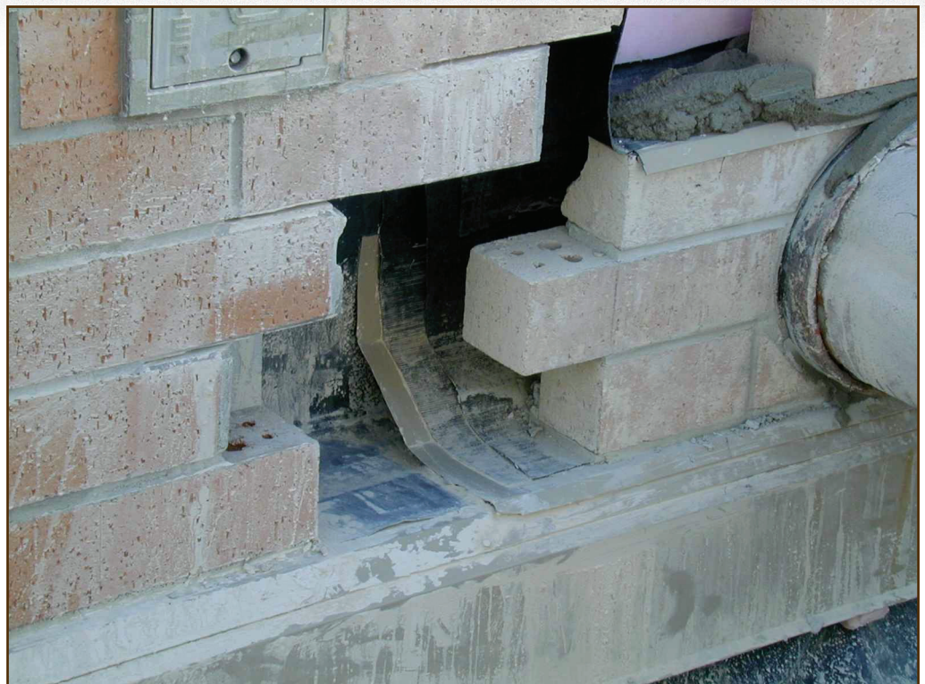
Figure 4 – Sagging initial through-wall flashing (under new metal flashing) creates an internal gutter that leaked.
