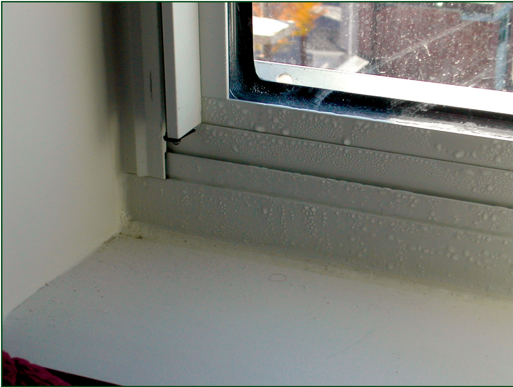
Left: Photo 2 – The installation of curtains (not shown) over this window led to significant condensation on the frame; the same window without interior curtains did not experience condensation.
