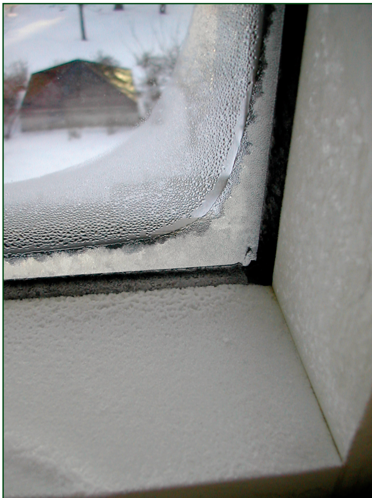
Photo 1 – Although selected for its high CRF, the installation method for this curtain wall caused significant thermal bridging around the frame, leading to condensation and even frost buildup on its interior surfaces.
