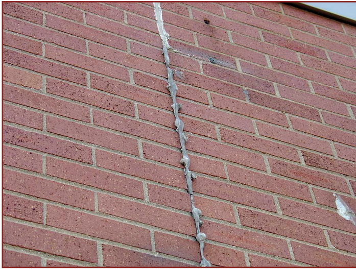
Photo 2: Sealant compressed out of improperly sized vertical expansion joint.
