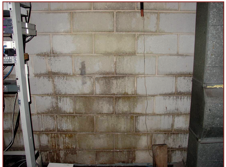
Photo 1: Water penetrating to interior surface of CMU wythe of solid masonry wall.
