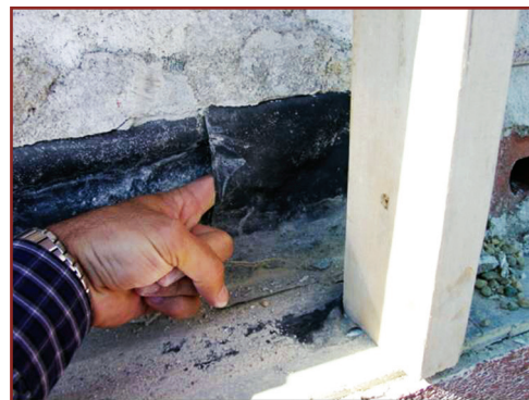
Photo 6: Improperly sealed flashing seam.
