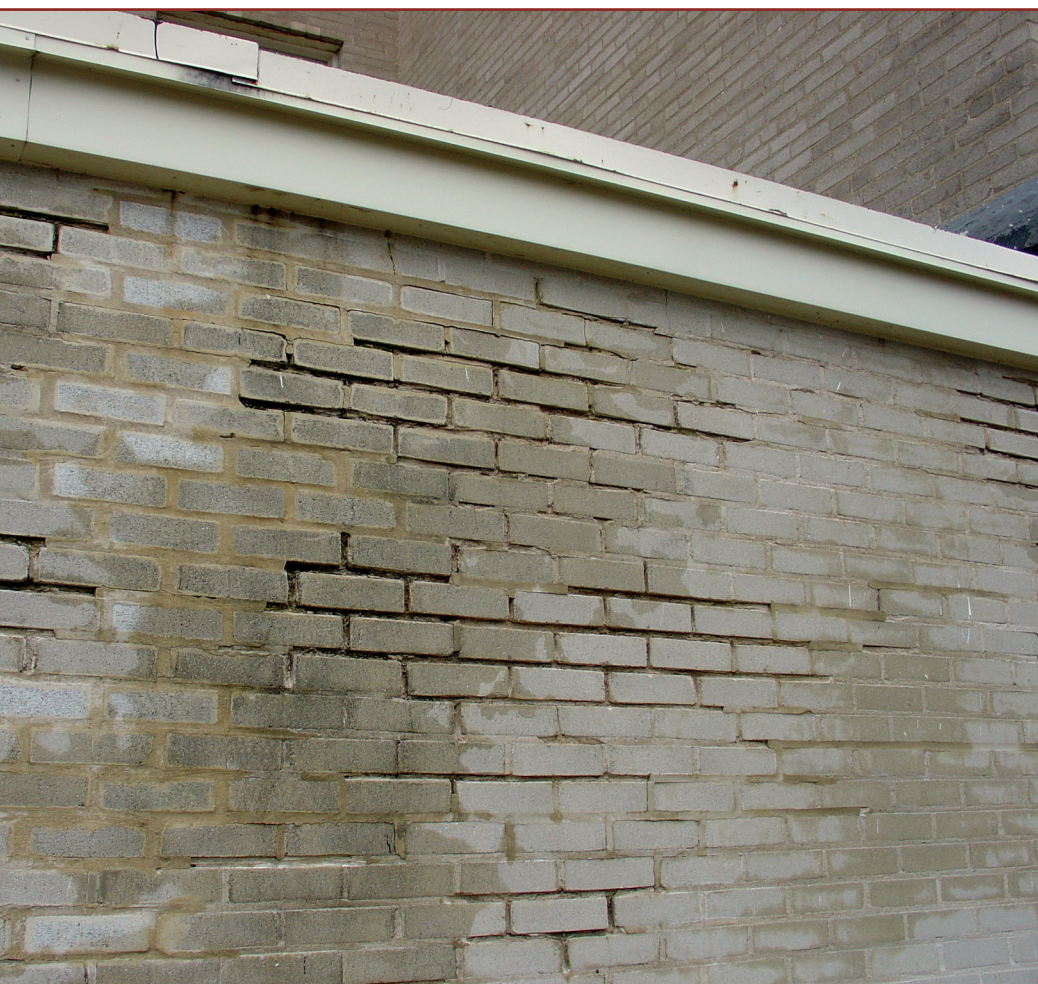
Photo 4: Freeze-thaw deteriorated mortar joints.
