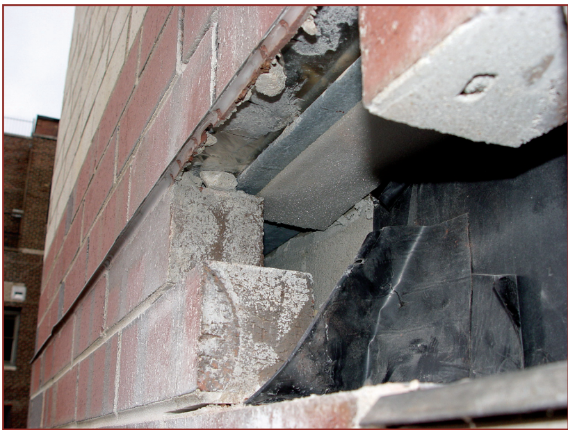
Photo 5: Mortar improperly placed in horizontal mortar joint and brick not properly supported on shelf angle.
