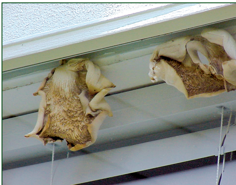
Photo 1: Previously undetected moisture is revealed through mushroom growth in a homeowner’s window.
