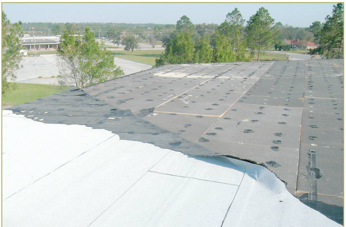
Figure 1: A built-up roof covering lifted and peeled back near one corner.
