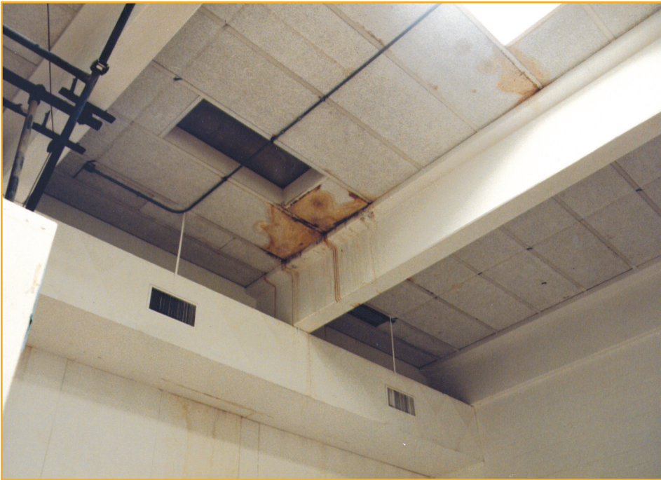
Apparent ceiling leak. (Photo courtesy Fincastle Engineering.)
