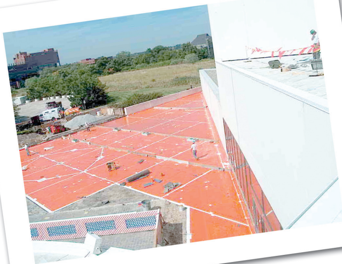
Photo 2 – The reinforced PVC waterproofing system was installed in a containment grid configuration to isolate any water that might breach the system.
