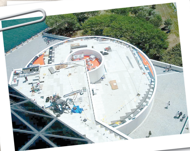
Photo 4 – Granite pavers were installed to complete the installation on the complexly-shaped elevated blue decks.
