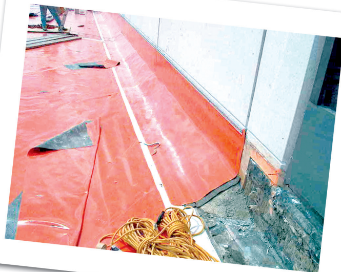
Photo 3 – A reglet was cut into the existing custom pre-cast concrete panels to terminate the waterproofing membrane and allow water to weep from the vertical caulk joints.
