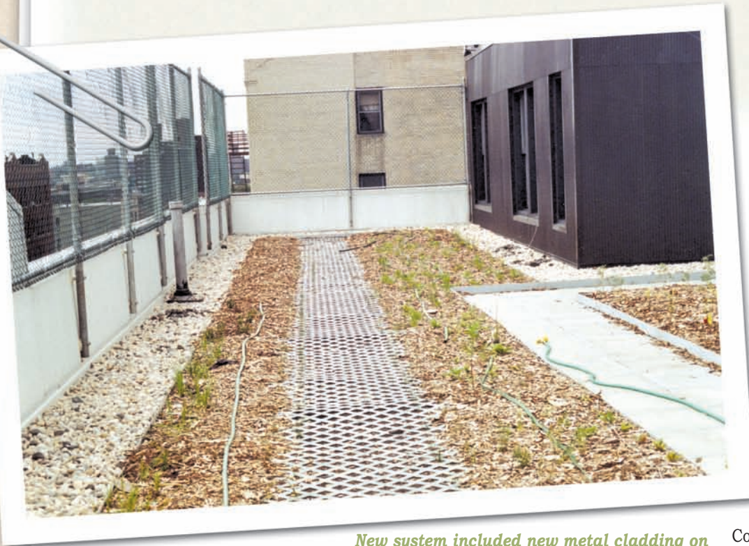
New system included new metal cladding on parapets and penthouses and safety fence at exterior parapets.
