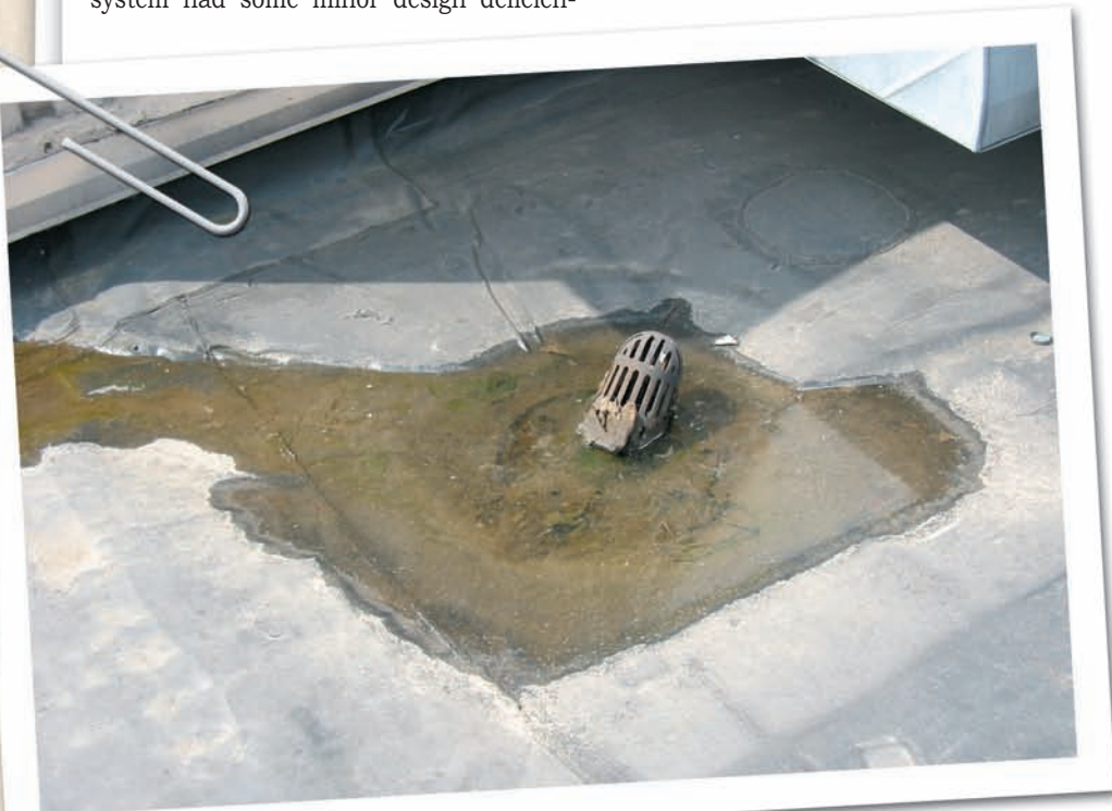
The drainage system and roofing membrane were found to be in need of restoration on the roof of the City of Milwaukee Northwest Garage.
