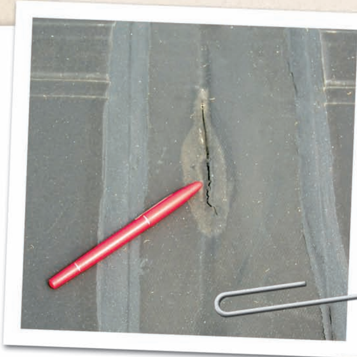
Separation of the seams of the EPDM roofing membrane were visible during inspection of the roof on the Milwaukee Northwest Garage.
