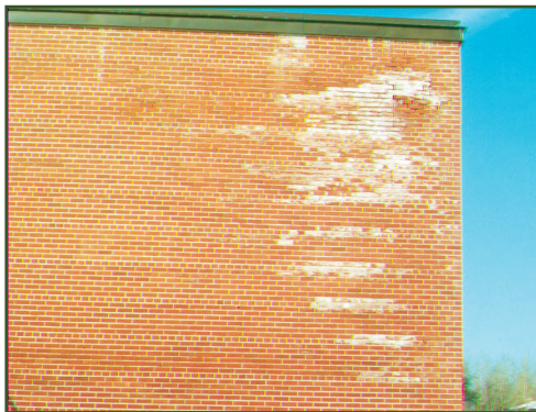
Building façade distress due to uncontrolled air leakage from the interior of a building in a cold climate.
