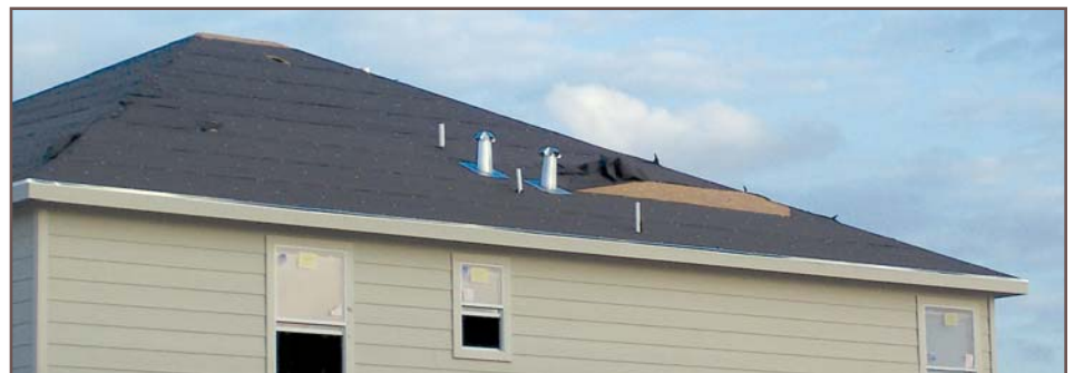
Felt underlayment displaced by wind.
