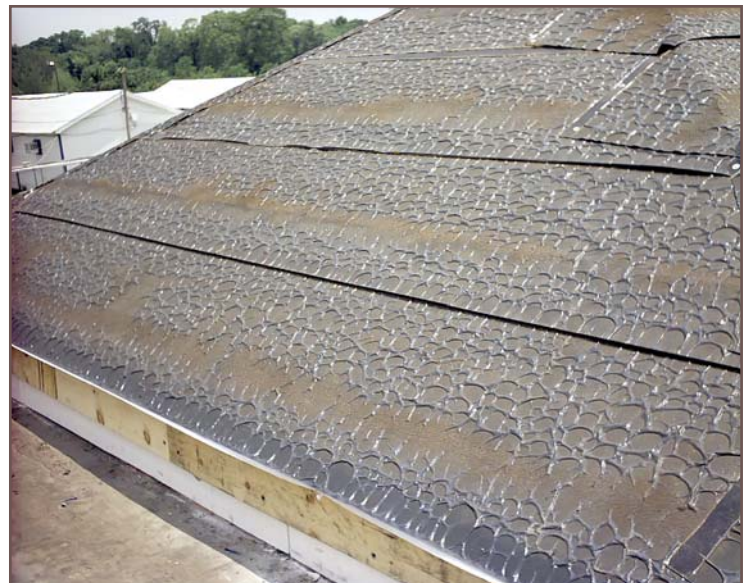
Wrinkled rubberized underlayment due to overexposure.
